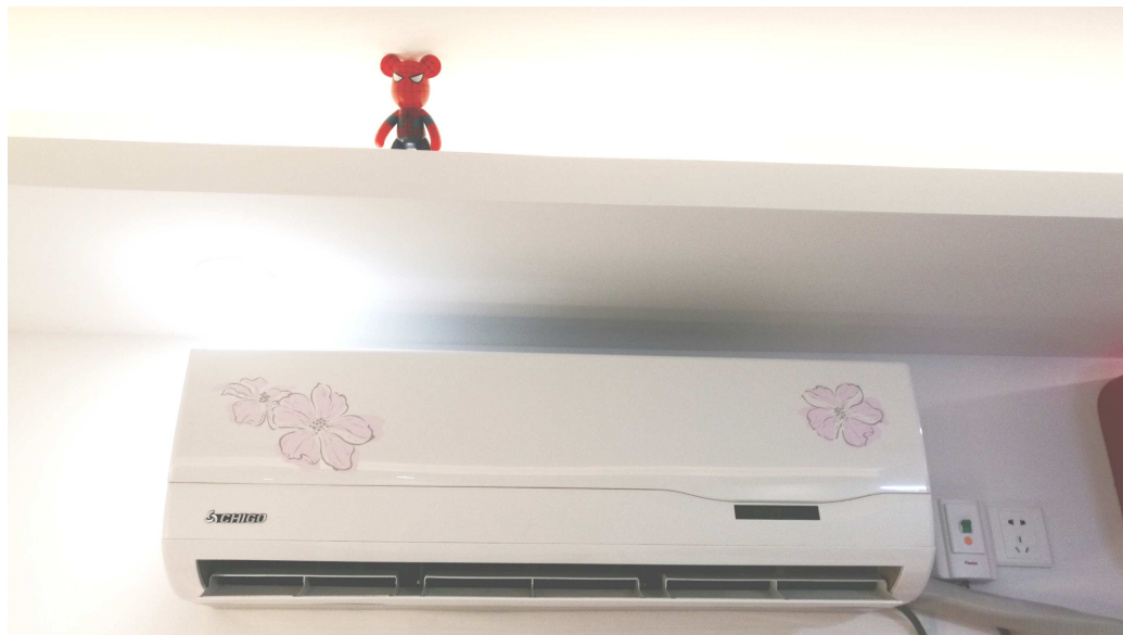
017 - Brand New ACs in all Rooms
