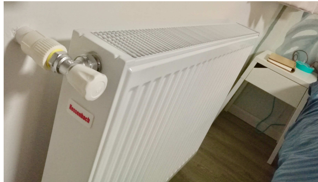
016 - Wall Heating in all Rooms
